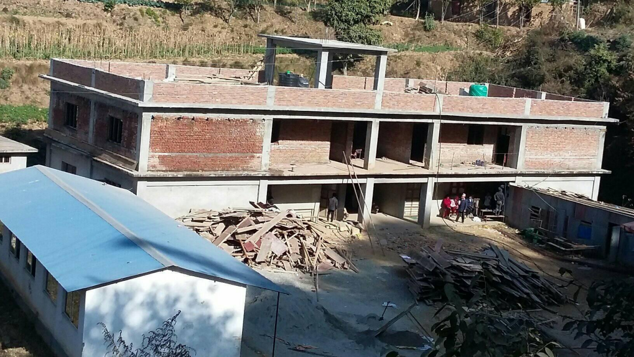
Nearly completed the project of rooms and rooftop with the materials we provided.
